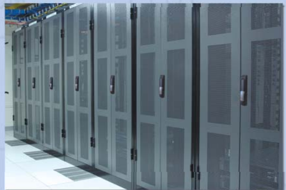
Access control at the server cabinets
