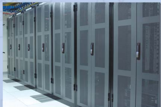
Access control at the server cabinets
