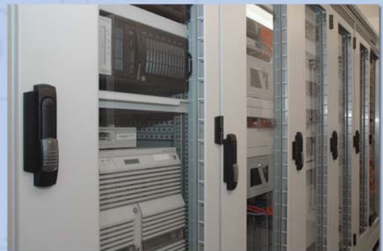
Access control at the server cabinets
