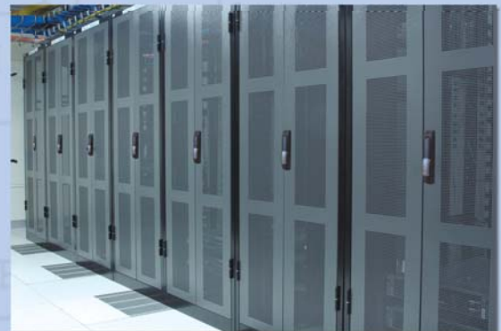
Access control at the server cabinets
