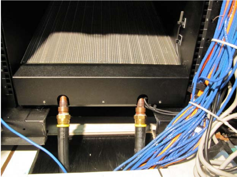
Bottom rear view of the CLWCE, showing the heat exchanger connections.
